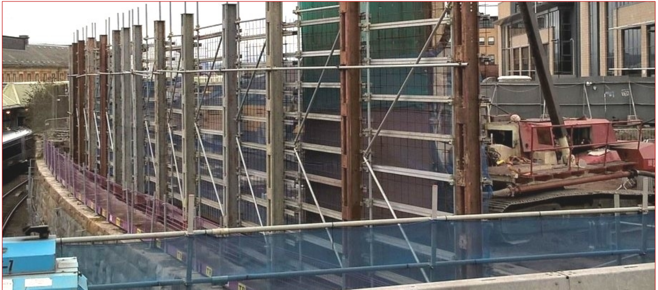
Piling immediately adjacent to the railway behind safety screens which permitted normal daytime working
