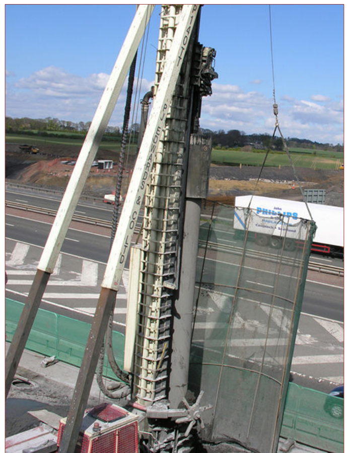
The P-140-TT Llamada Rig in DTHH mode with safety screen suspended from the rig to protect passing traffic
